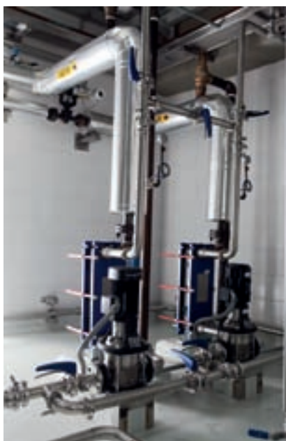
Washer – dryer system #4, the Colcafé Plant; Medellín, Colombia.
