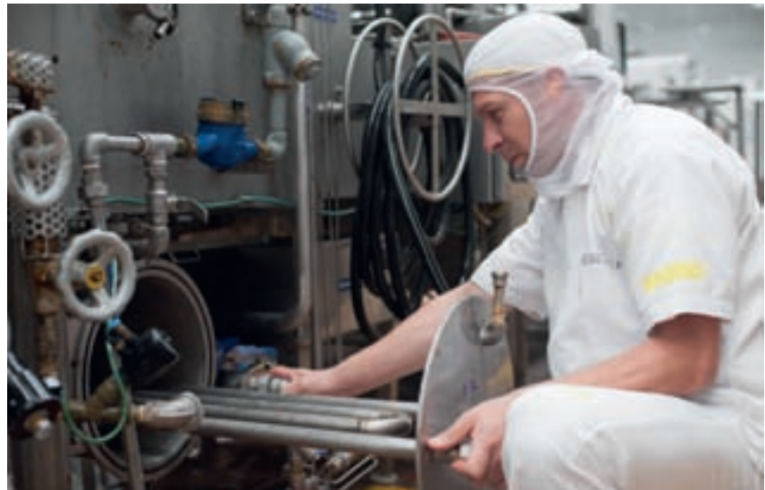
Heating coils in the demolding tank, Meals de Colombia Plant; Bogotá, Colombia.
