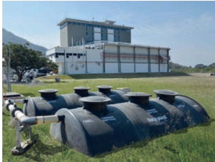
The wastewater – treatment plant, Molino Santa Marta ; Santa Marta, Colombia.
