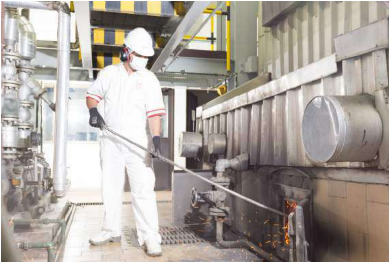
Steam generator that uses biomass from the soluble coffee extraction process, Coffee Business, Colombia.
