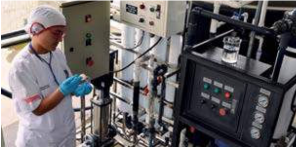
Recovered Water Treatment System for industrial services, Pastas Doria. Mosquera, Colombia.
